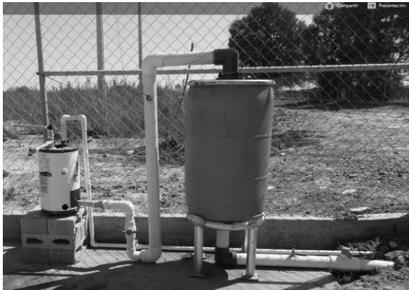
Fig. 5. Image of the Test Bench # 1 (BE-1)
